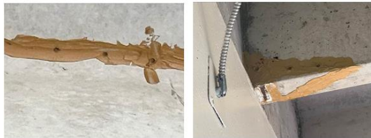
Example of past repairs to the flanges and stems of the precast concrete double tees
