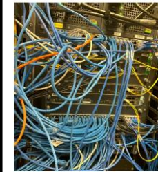
MDF Patch panels and Electronics
