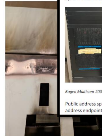
Figure 3 Switchboard 2 Fire Damage
