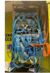
IDF Patch Panels and Electronics
