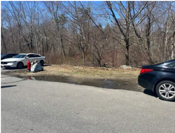
Figure 15 – West Site Ponding
