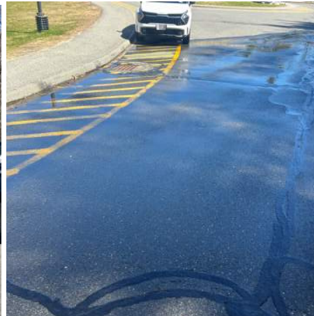
Figure 16 – Ponding at SW
