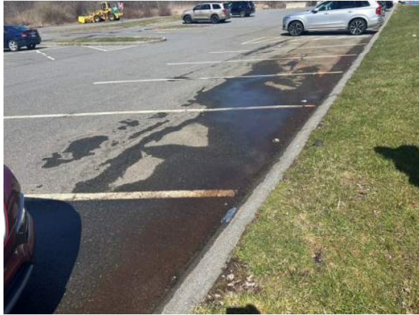
Figure 18 – Ponding at Northern Parking Lot
