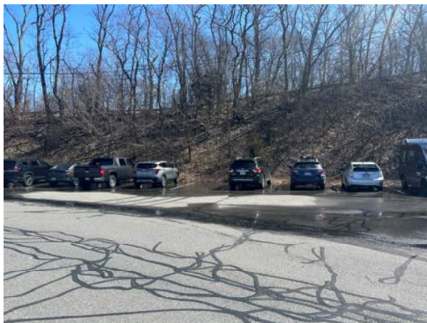
Figure 20 – Ponding at South Parking Lot
