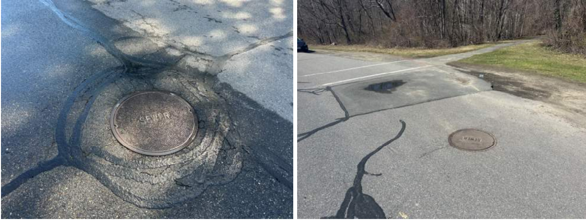
Figures 12 and 13 - Sewer Manholes on the Southwest and West Side of the Building
