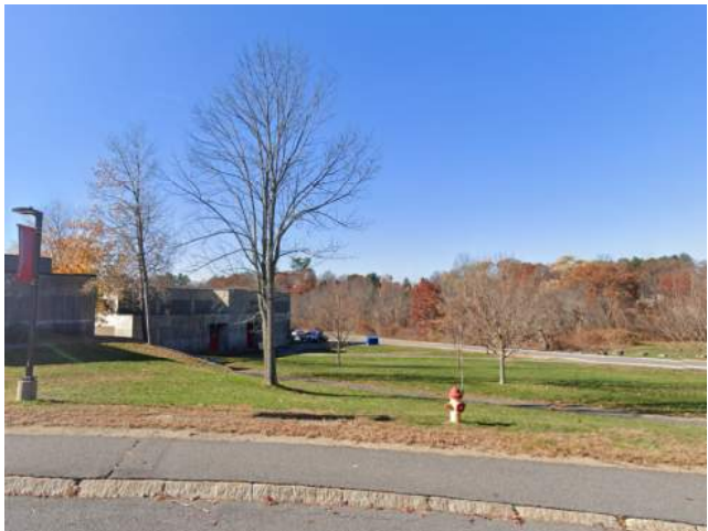
Figure 10: Hydrant at Turnaround
