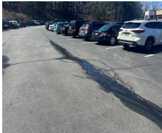
Figure 21 – Ponding at South Parking Lot
