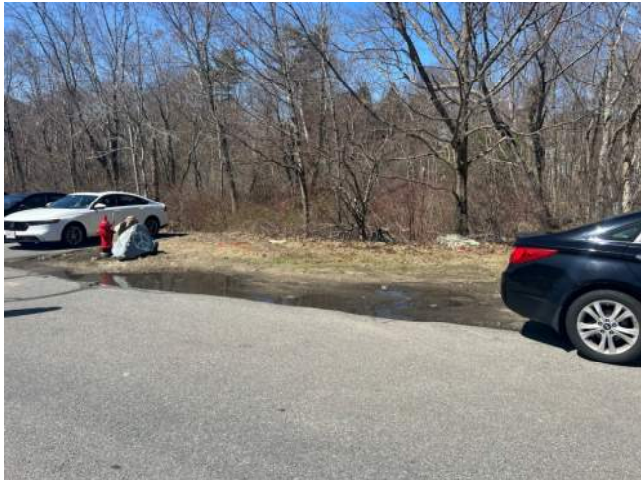
Figure 8: Hydrant West of Building
