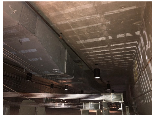
Photo 4- Sprinklers above Stage
