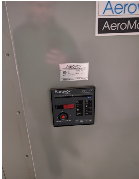
Figure 2 Power Factor Correction unit SWBD 1 , dated 1994.
