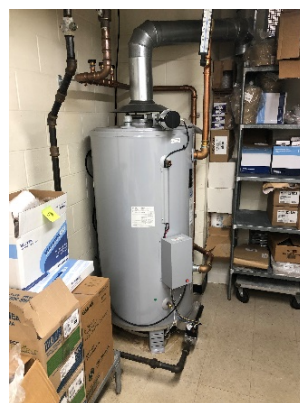
Photo 8 – Kitchen Water Heater
