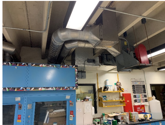
Photo 4 – Exhaust Hood with Make-up Air Fan
