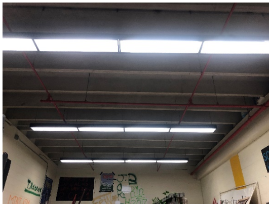
Photo 3 – Storage Room Sprinklers
