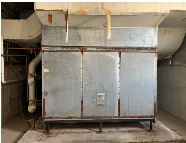
Photo 6 – Penthouse Air Handling Unit
