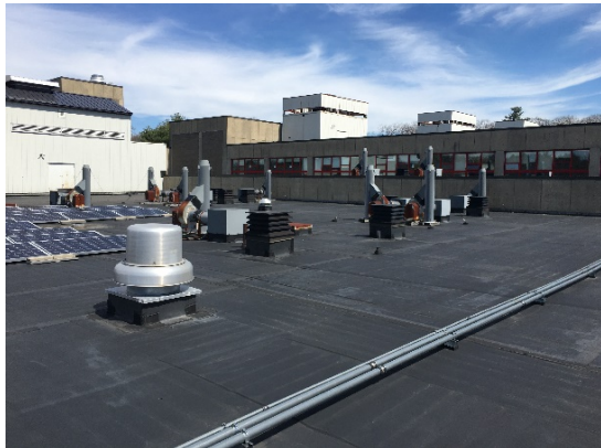
Photo 3 – Rooftop Exhaust Fans
