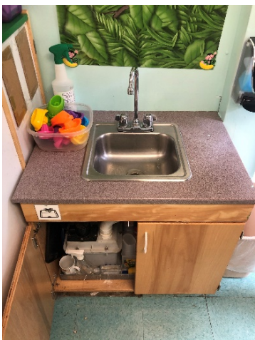
Classroom Sink with Drain Pump
