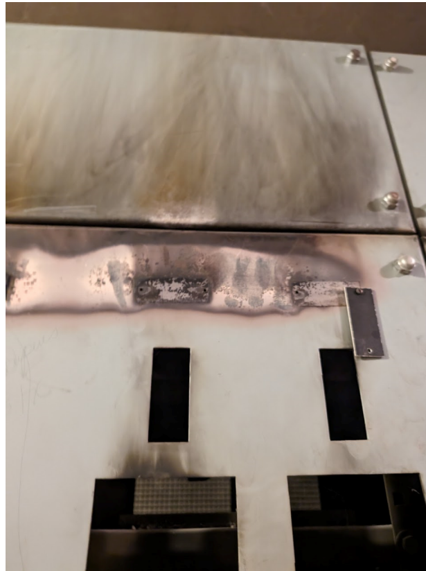
Figure 3 Switchboard 2 Fire Damage
