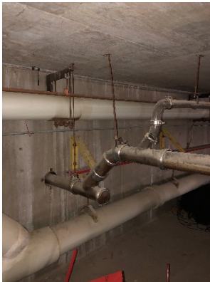
Photo 11 – Glass Waste Piping
