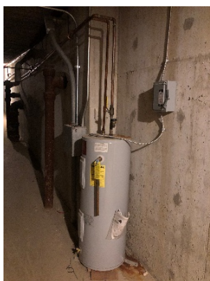
Photo 7 – Electric Water Heater
