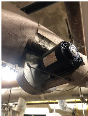
Photo 5 – Draft Inducer Fan
